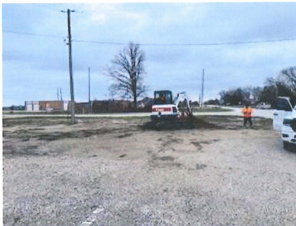
PHOTO 4 – EXCAVATION OF TEST PITS IN THE AREA OF THE EXISTING CONCRETE PAD – WEST
