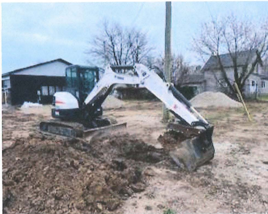
PHOTO 3 – EXCAVATION OF TEST PITS IN THE AREA OF THE EXISTING CONCRETE PAD – SOUTH
