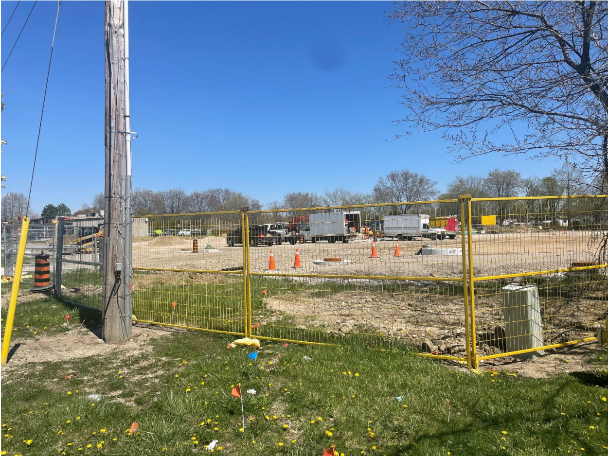
Photo 4: Taken from Sandwich St. S. facing north-east. The photo shows the on-going construction on the site.
